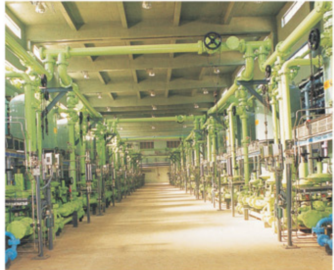
O & M services at power station
