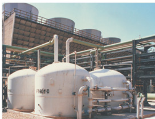
Cooling water treatment
