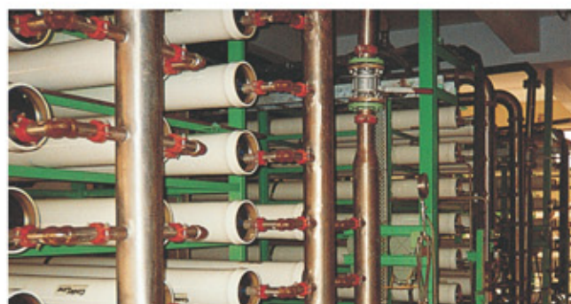
Zero discharge plant
