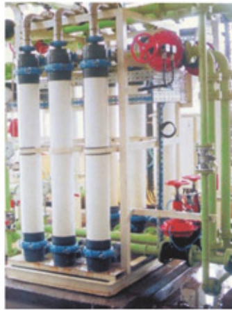
Ultra filtration plant
