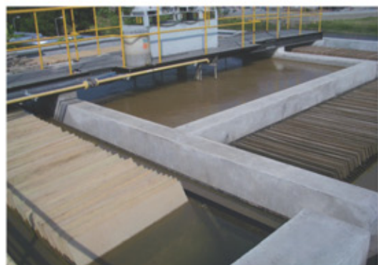
Ultra high rate clarifier
