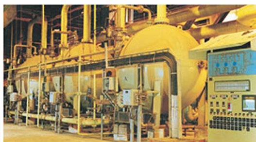
Condensate polishing units
