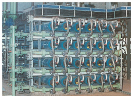
Sea water reverse osmosis desalination plant
